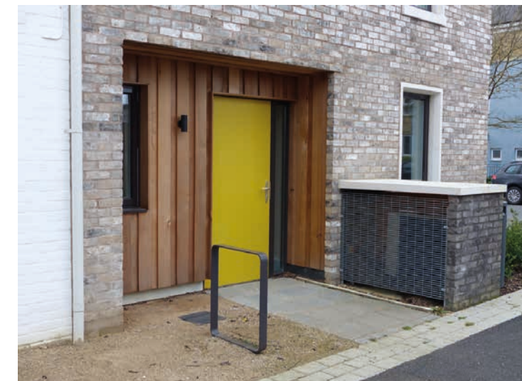
Example of a well concealed air source heat pump. Marmalade Lane, Cambridge
